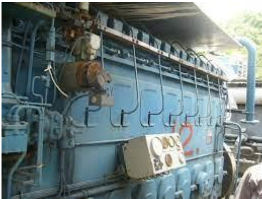
L 20/27 Diesel motor.
